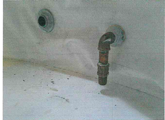
Pictured is the 2" outlet and 1" drain/test line.
