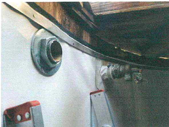
Pictured is the 2" overflow and inlet.
