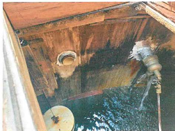
2" pipe inlet & overflow
