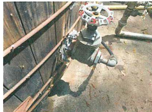
4" flange outlet/test port
